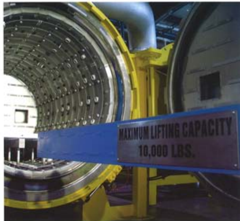
Dedicated Powered Load Truck in use at Solar Atmospheres, Souderton, PA.
